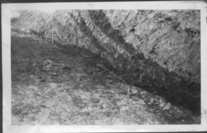
Bourne South Fen New Pumping Station. Sections showing peat strata of River Glen Bank.
