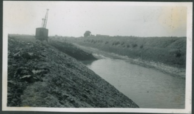
South Drove Drain, Improvement 1948. Work in progress between Horseshoe Bridge and 2 nd Railway Bridge.
