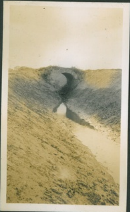
SLIGHT UN-ALIGNMENT OF EXISTING STONE BRIDGE.
