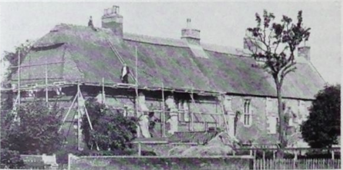
An old photograph by Stanley Jepson showing the thatching of the buildings built out of priory remains. The thatching surface covers 5,000 square feet, the thatch was 20 inches thick and 1,000 bundles of reed were used in what is believed to be the largest thatched surface in England. The work took eight weeks.
